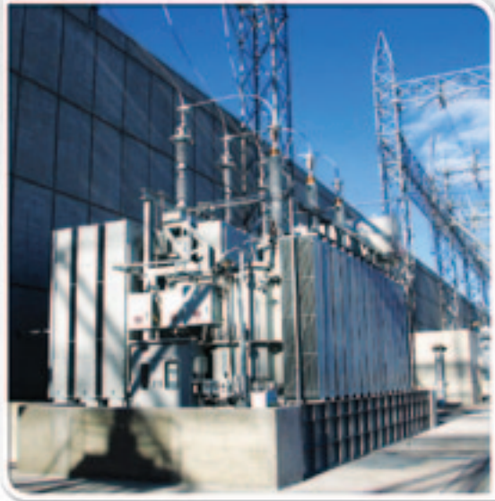
Fig.3 Application of FO sensor for cooling control on 240 MVA transformer at GCPUD.
